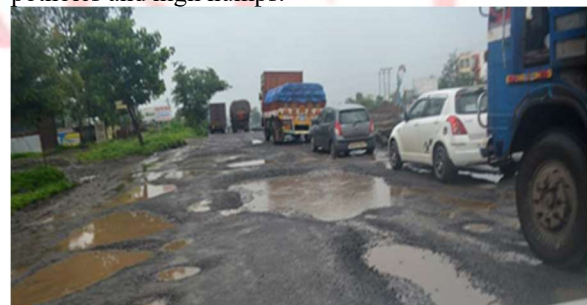
Fig. 1 potholes on roads that are a death trap
